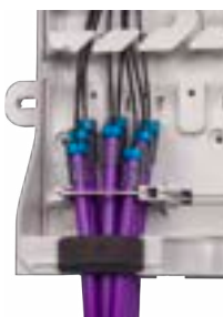
Microduct Termination in the Box
