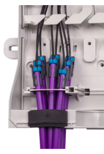
Microduct Termination in the Box
