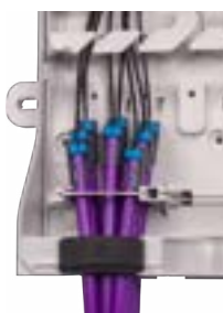
Microduct Termination in the Box
